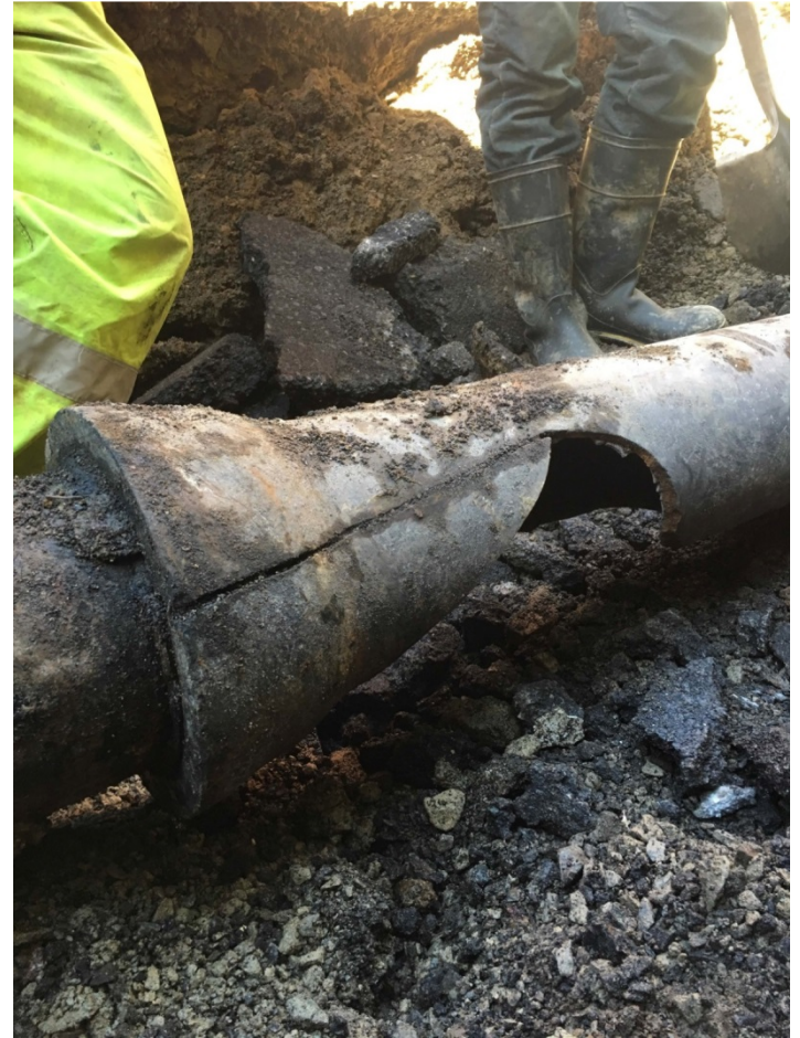
Leak on 65 year old cast iron pipe in Fairfax (June 10 th )
